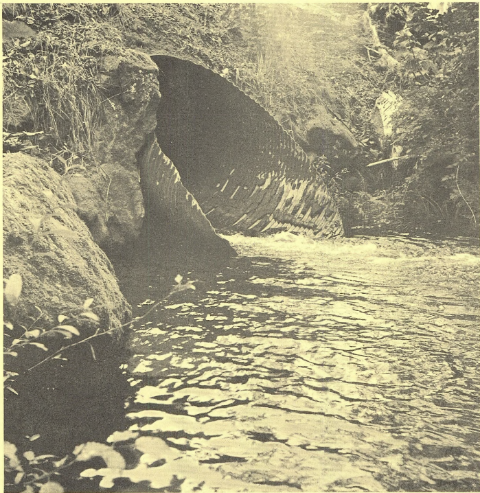
Illustration 5 - GOLD CREEK - Culvert outlet after dams were built.
